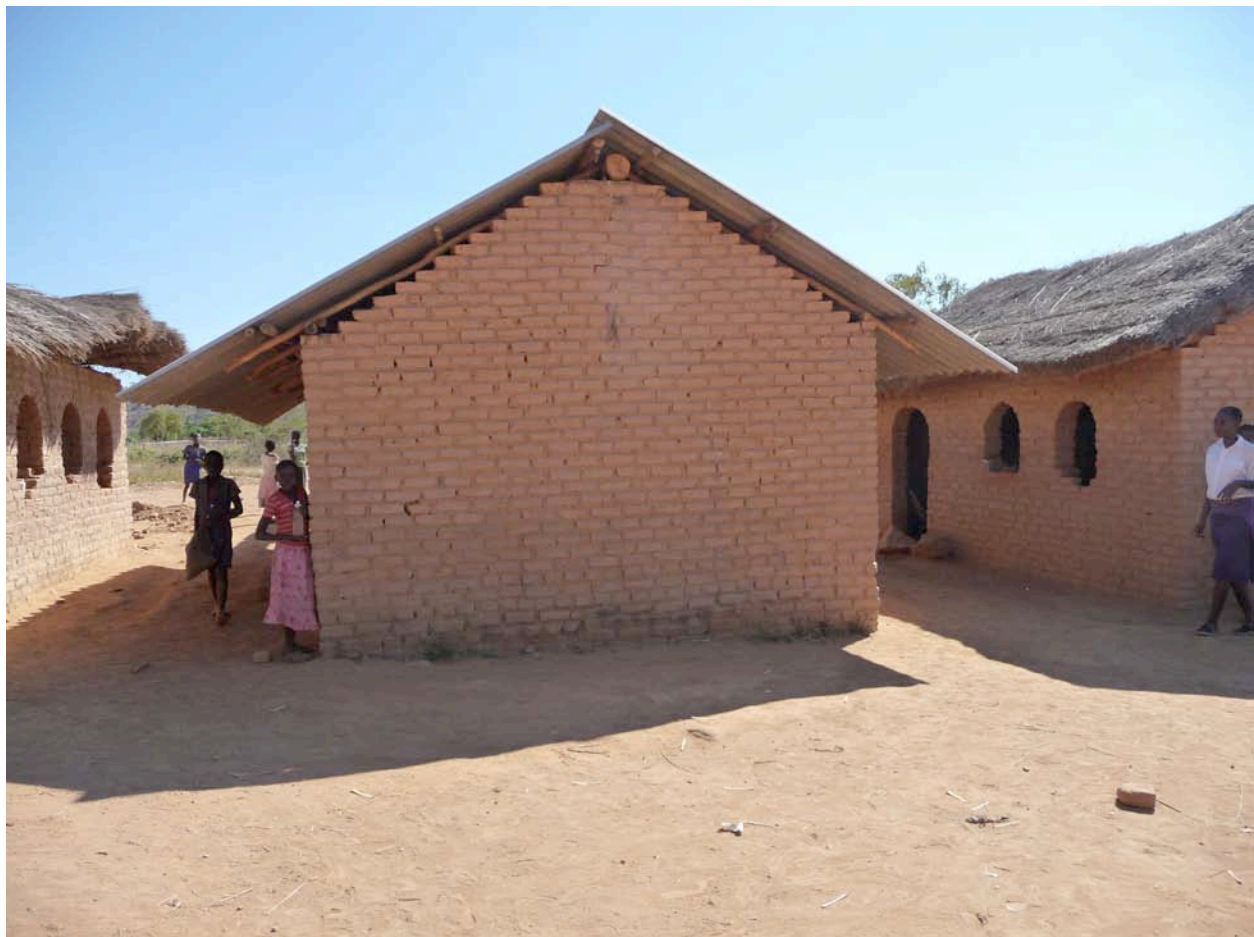
New rooves for some of the classrooms at Obert's school have already been constructed
